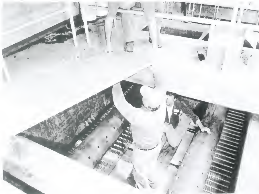
Rehabilitation of the Water Treatment Plant clarifier by DPW staff Skip McEvoy, Dick Rowe & Ed Bugbee - May 2007
